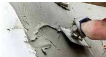
DryMix Building Materials Processing
